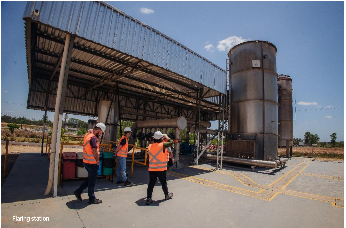
Three main lines of landfill gas coming into the flaring station.
